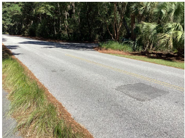
Pavement overview – Note vehicular stains
