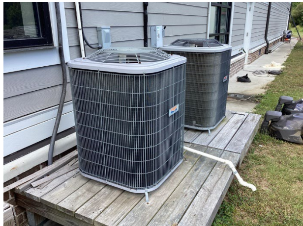
Split system condensing units at maintenance building
