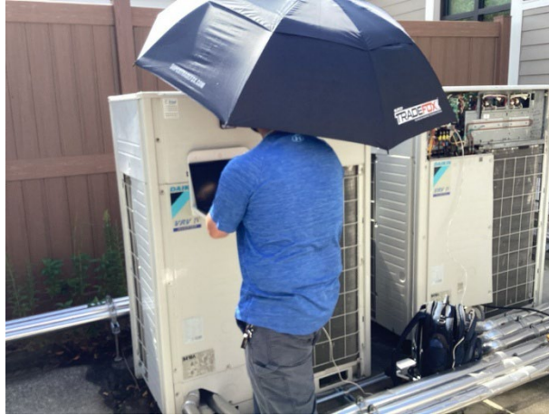
Outdoor heat pump units
