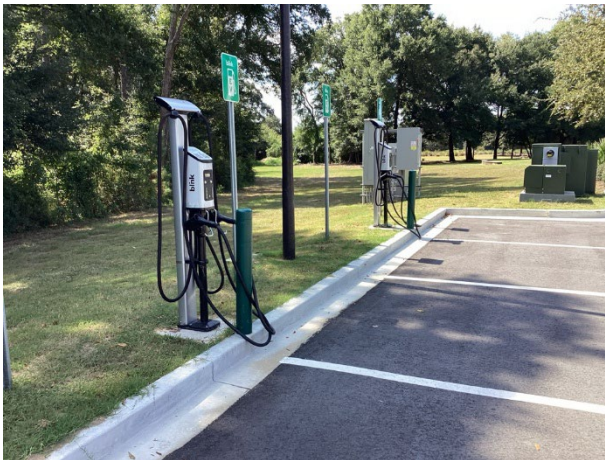
EV Charging station equipment
