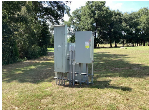
EV Charging station equipment
