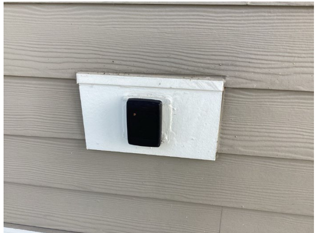
Access control point
