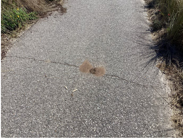
Walking path cracks
