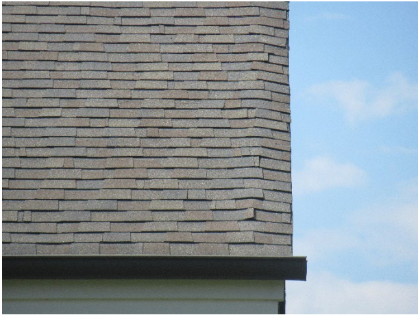
Asphalt shingle roof overview – Note shingle curl
