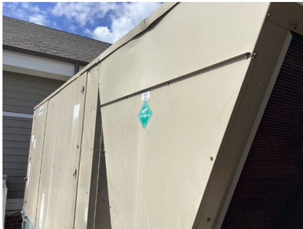
Make-up air unit
