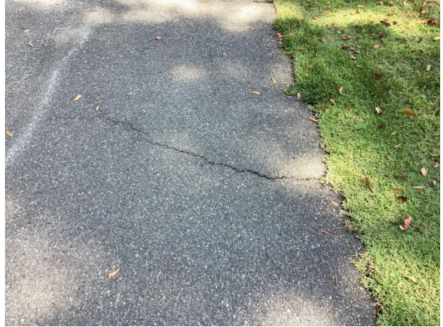
Walking path cracks
