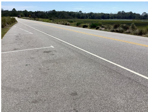
Pavement overview – Note vehicular stains
