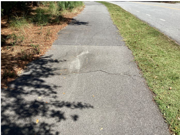
Walking path cracks
