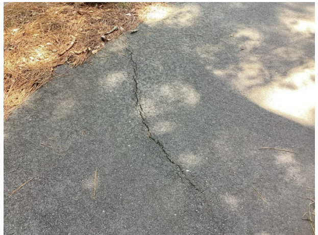
Walking path cracks
